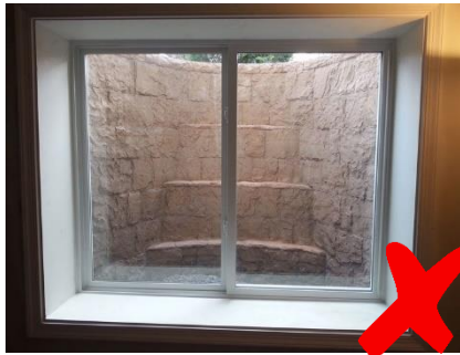
Does not show where/which room egress is located
